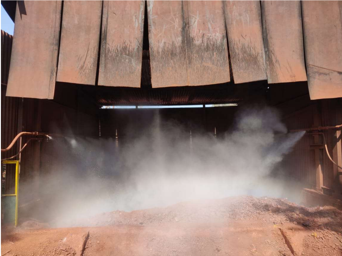
PHOTO: 7 PHOTOGRAPH SHOWING DRY FOG SYSTEM IN OPERATION
