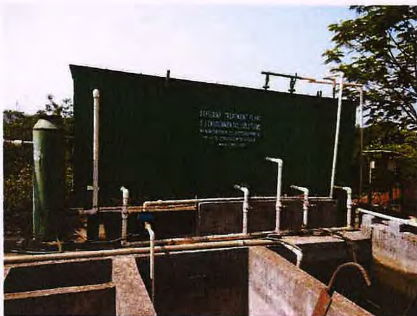
PHOTOGRAPH OF ETP
