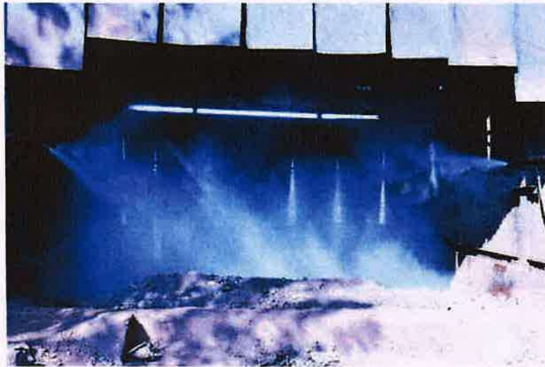
DRY FOG SYSTEM IN WORK
