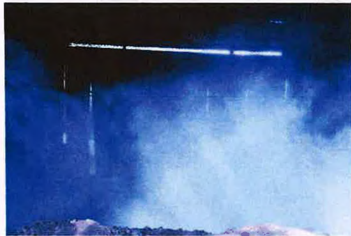
DRY FOG SYSTEM IN CRUSHING UNIT
