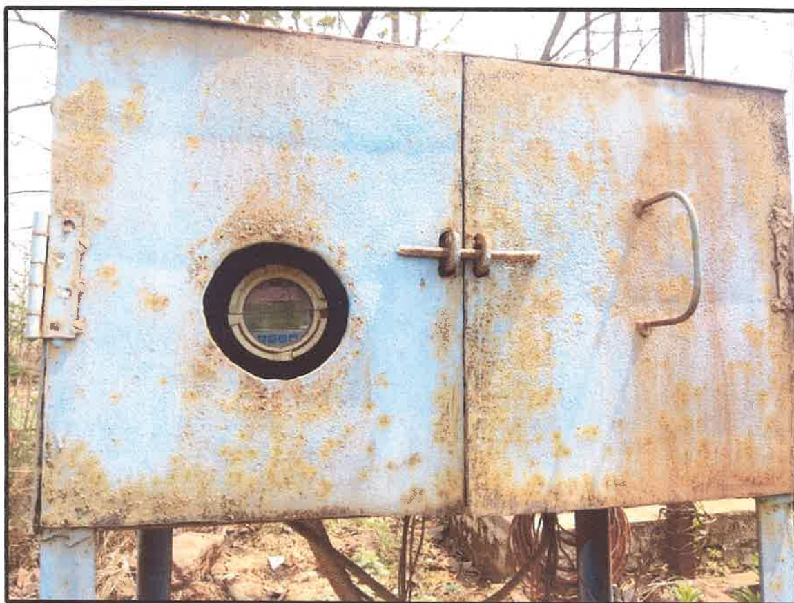
PHOTOGRAPH OF DIGITAL FLOWMETER
