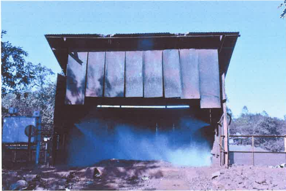
DRY FOG SYSTEM IN SCREENING UNIT
