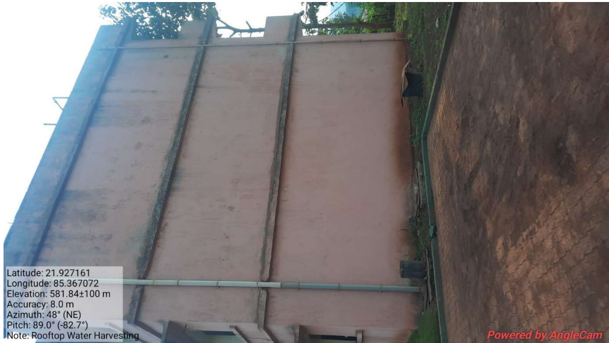
PHOTOGRAPH OF ROOFTOP WATER HARVESTING PIPELINE
