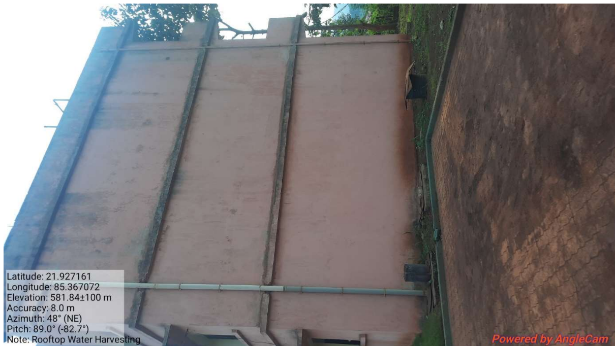
PHOTOGRAPH OF ROOFTOP WATER HARVESTING PIPELINE
